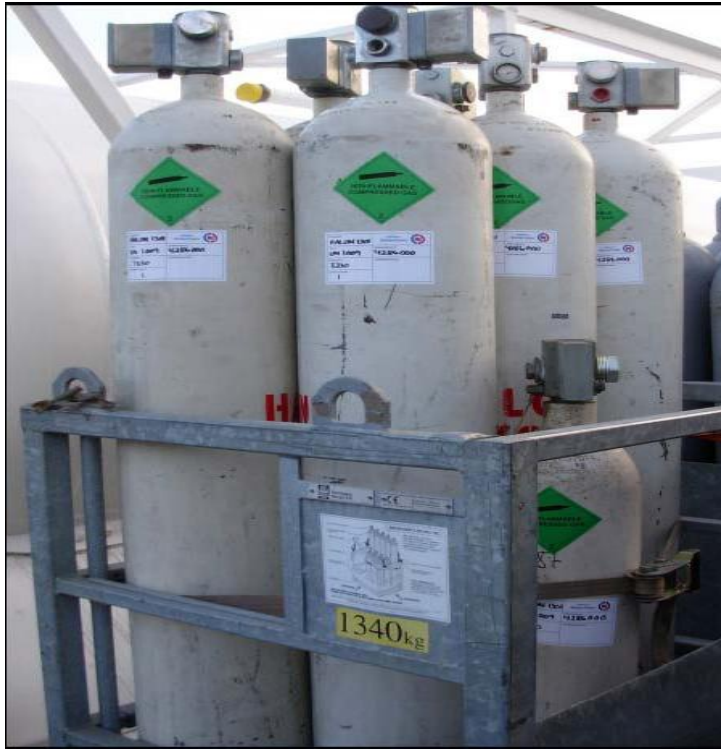
Picture 3. Correct labeling and packing of halon cylinders.
