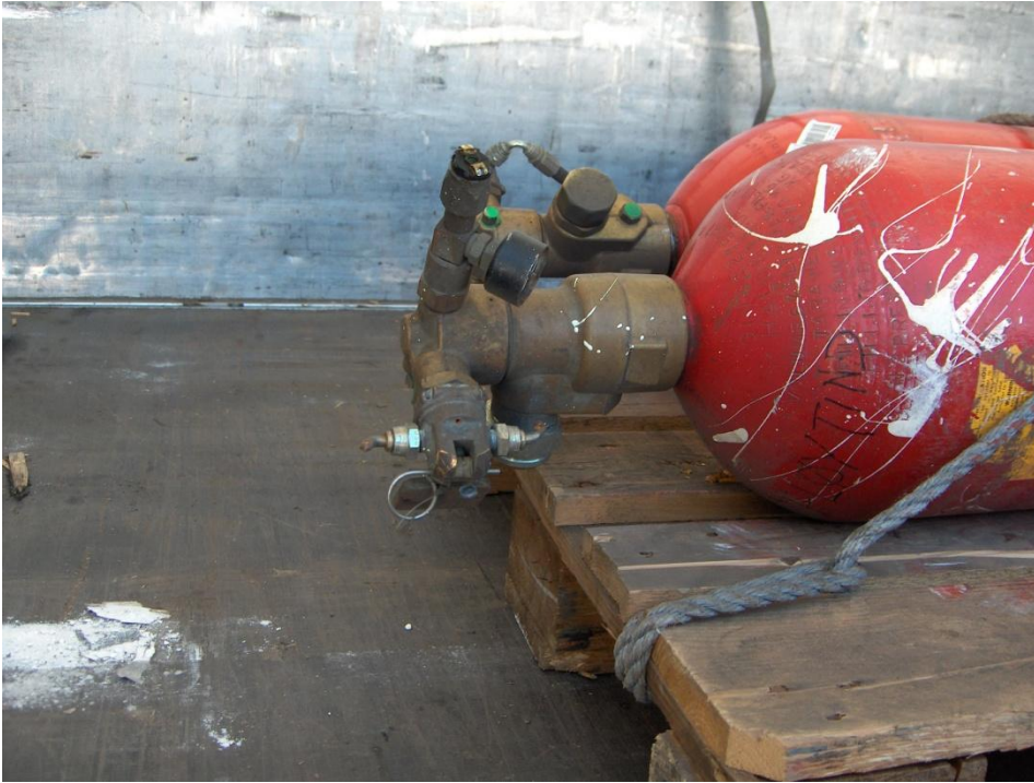
Picture 5. Unprotected valves
